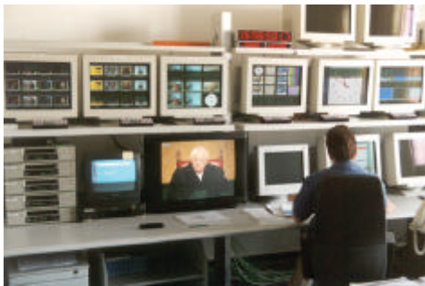
Quality control and monitoring of the satellite transponder parameter takes place in the Network Management department
