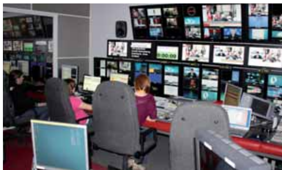
Studio control: Cabling started early March 2008 along with the installation of racks, air-conditioning and furniture
