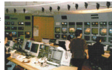
VTRs have been moved back into the control desk area
